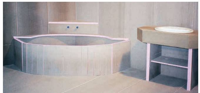
Beautifully designed washstands are as simple to create as the cladding for bathroom walls.
