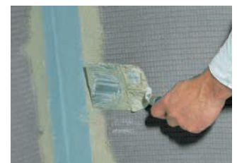
Then insert the sealing tape, fill it using wall leveller and the smooth substrate is ready.
